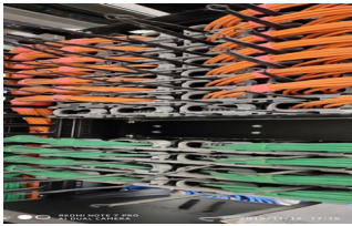
Shakthi Precision BMS Project - Networking
