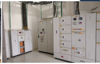
DCX Project Bangalore - LT Panels
