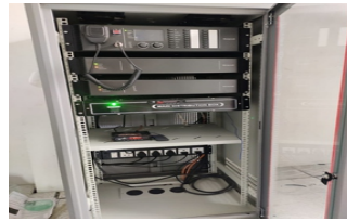
Shakthi Precision BMS Project - Public Addressable system
