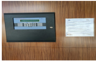
Shakthi Precision BMS Project - Fire Alarm System
