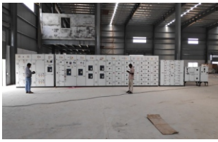
Time Technoplast Malur Project :- LT Panel
