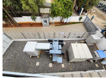
Applied Materils HT Yard
