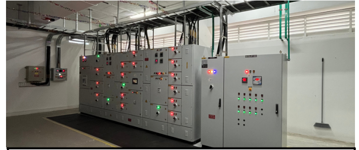
HT & LT DISTRIBUTION PANELS
