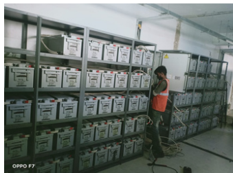
GEA Westfalia UPS/Battery Bank Connectivity
