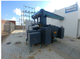
Bismi Ramnad 1600KVA HT yard
