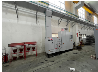
IBEX Engineering 1600A Bus Duct & LT Panel
