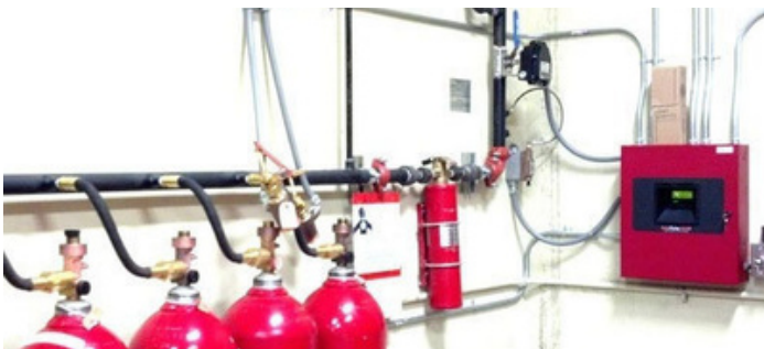
GAS SUPPRESSION SYSTEM
