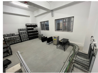
Homag UPS/Battery Bank Connectivity
