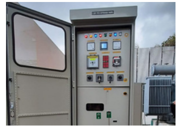
Shakti Precision 11KV VCB Panel
