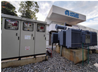
Applied Materials 2000KVA HT Yard
