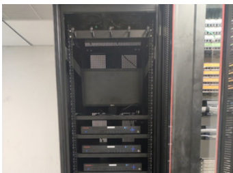
Shakti Precision IP CCTV Server Rack
