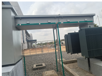
Meyer Organics 3000KVA HT Yard
