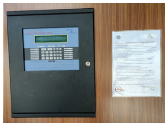
Shakti Precision Fire Alarm System
