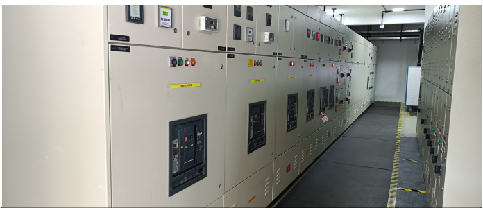
LT PANELS MANUFACTURING
