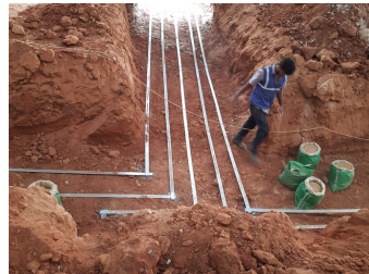
ABB Hitachi Substation Mat Earthing
