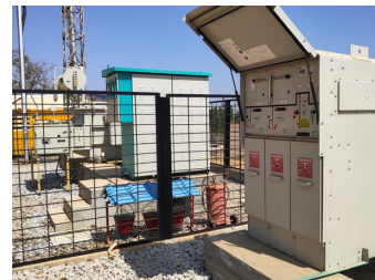
Rajdhani industrial Park 11KV RMU & Substation
