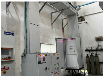
IBEX Engineering 1600A Bus Duct & LT Panel
